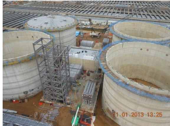
Fig. 1: Blue Plains Advanced Wastewater Treatment Plant aside the Potomac River
